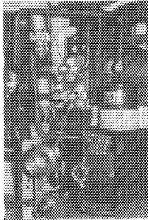
Stop valve at hot gas bypass
